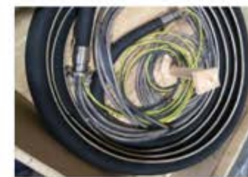
Service Loop - Power 2.jpg
